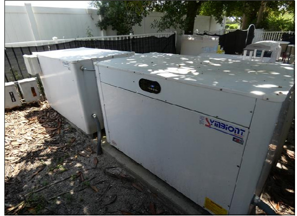
Swim Club Geothermal Heating Units
