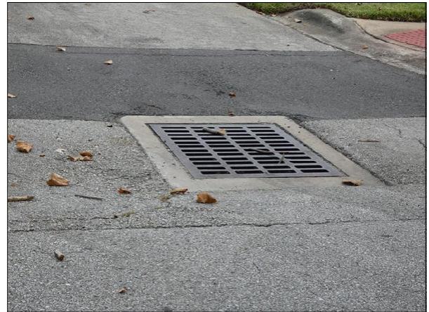
Stormwater Drainage Grate Inlet
