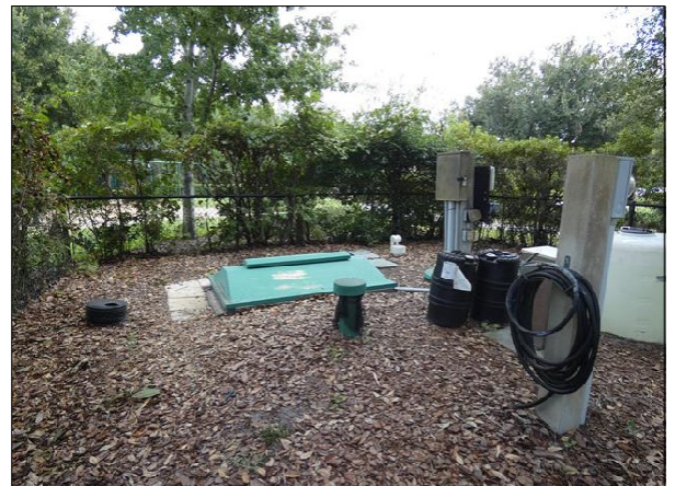
Lake Recreation Area Splash Pad Equipment
