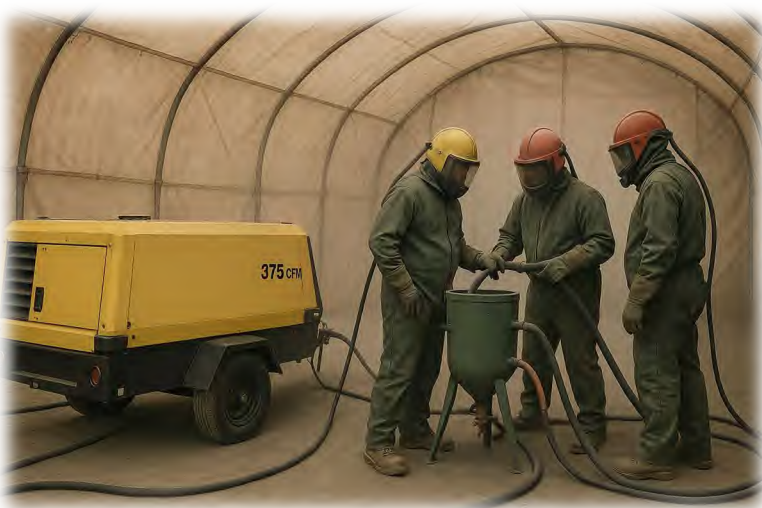
375CFM Compressor / Sand-Blast Equipment's
