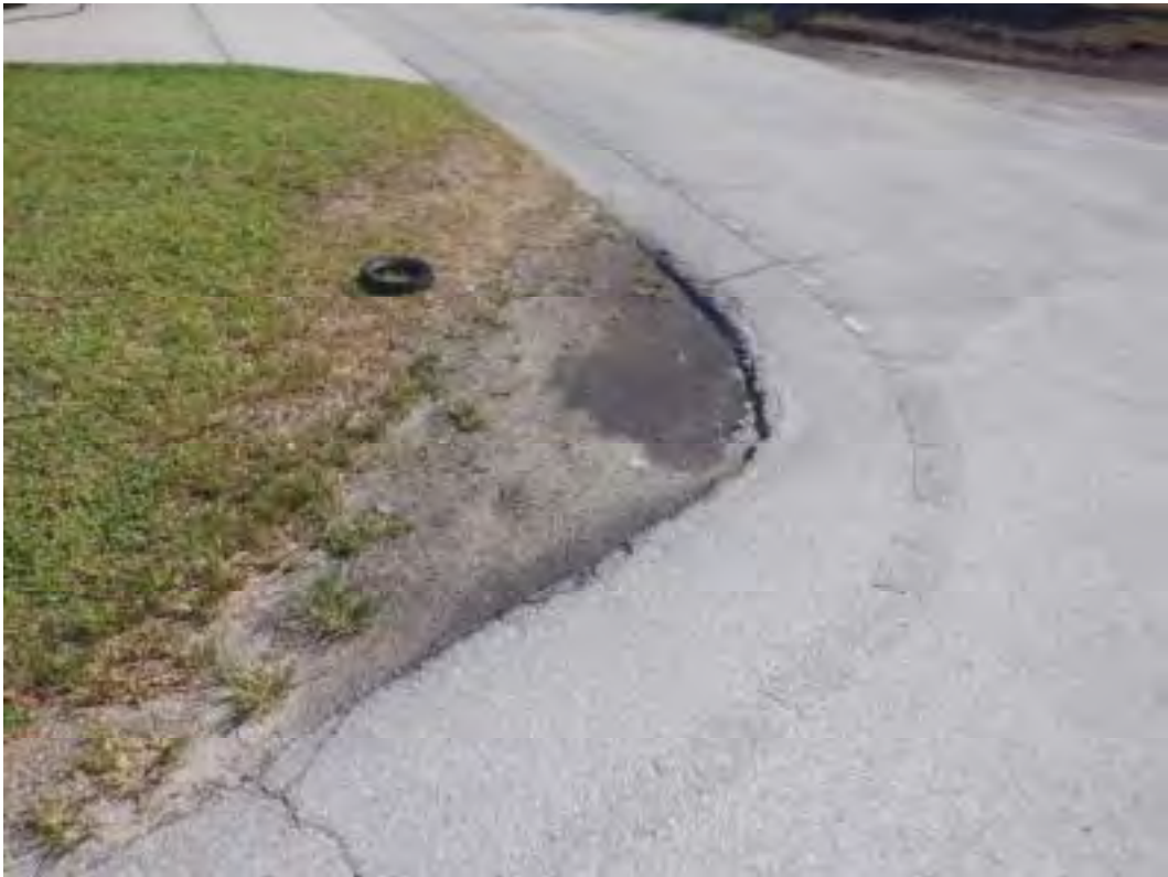
13-Alley road Date Taken: 6/7/2024 View of worn area
