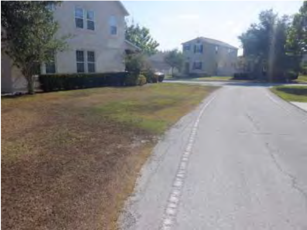
40-Alley Road Date Taken: 6/7/2024 View of reported damaged to sod area near damaged road
