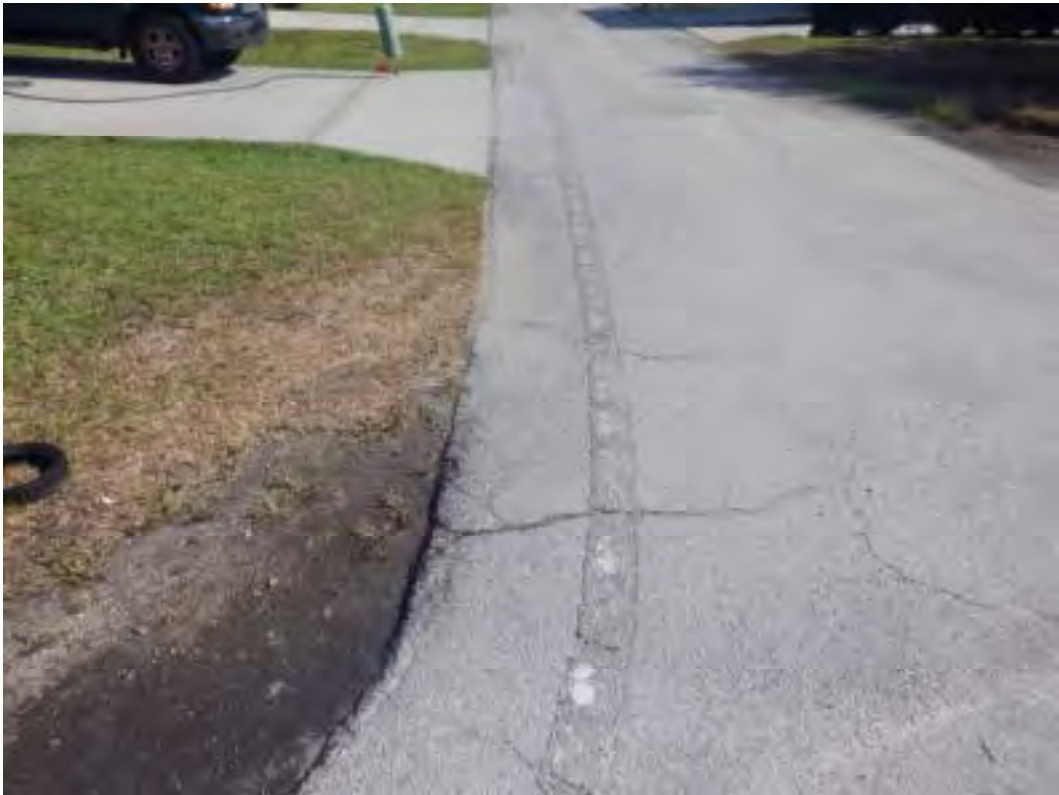
15-Alley road Date Taken: 6/7/2024 View of worn area
