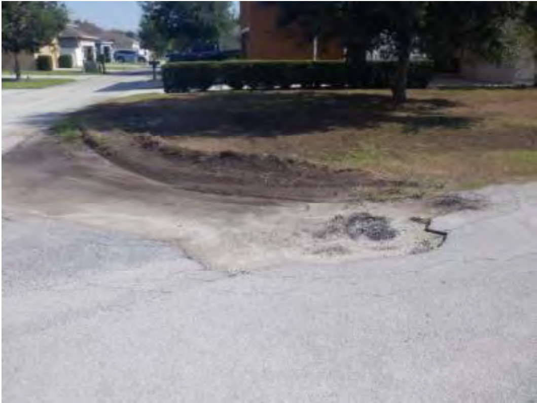
42-Alley Road Date Taken: 6/7/2024 View of reported damaged to sod area near damaged road
