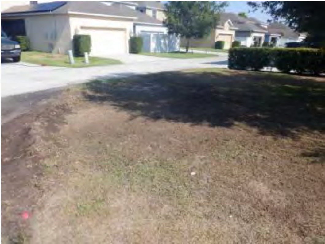
37-Alley Road Date Taken: 6/7/2024 View of reported damaged to sod area near damaged road
