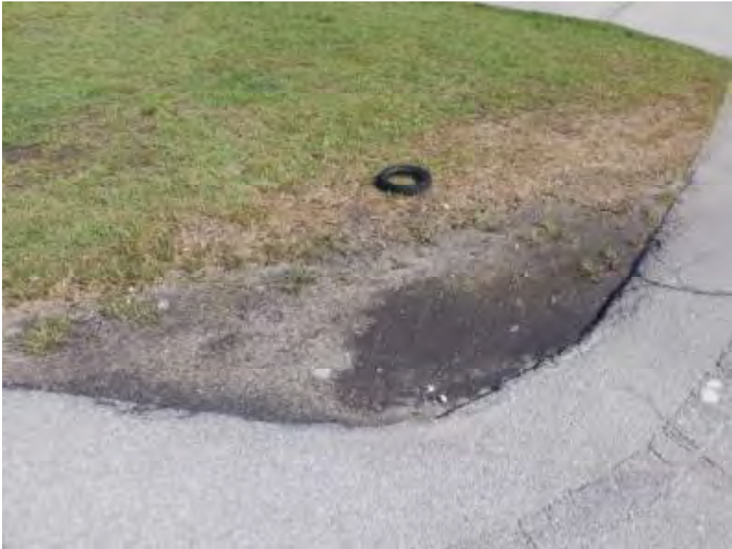
14-Alley road Date Taken: 6/7/2024 View of worn area
