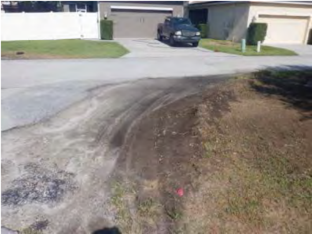
41-Alley Road Date Taken: 6/7/2024 View of reported damaged to sod area near damaged road
