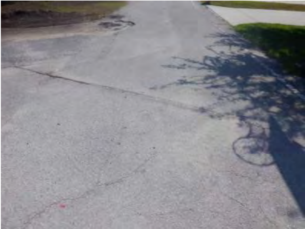
16-Alley Road Date Taken: 6/7/2024 View of road reported damaged by insured vehicle, age, deterioration, and/or wear & tear noticed to this area
